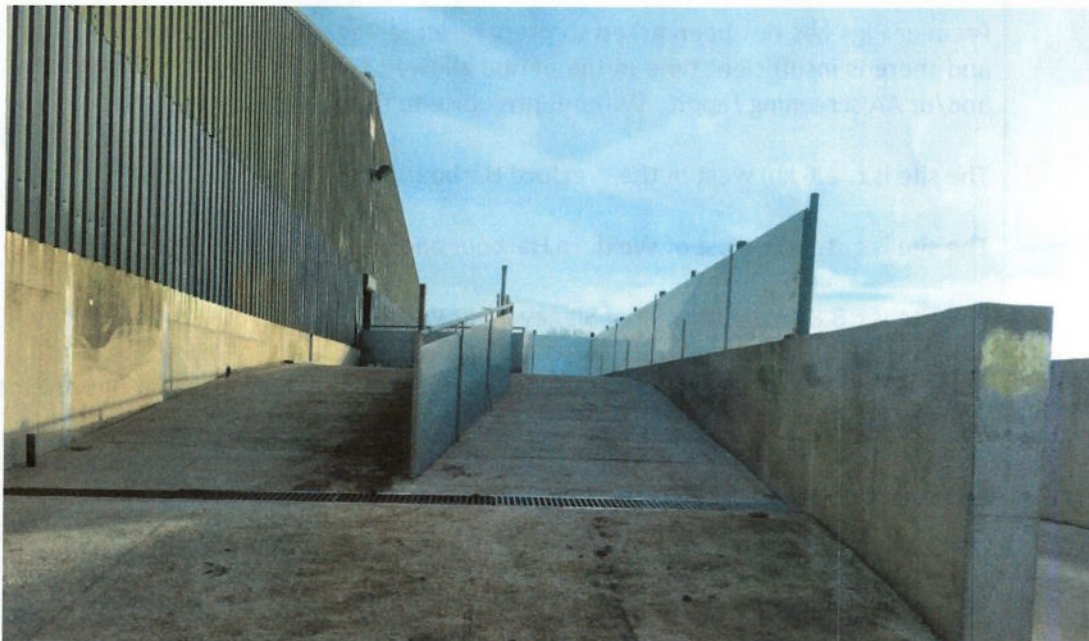
Figure 2: Photo showing that the ramp is attached to the shed.
